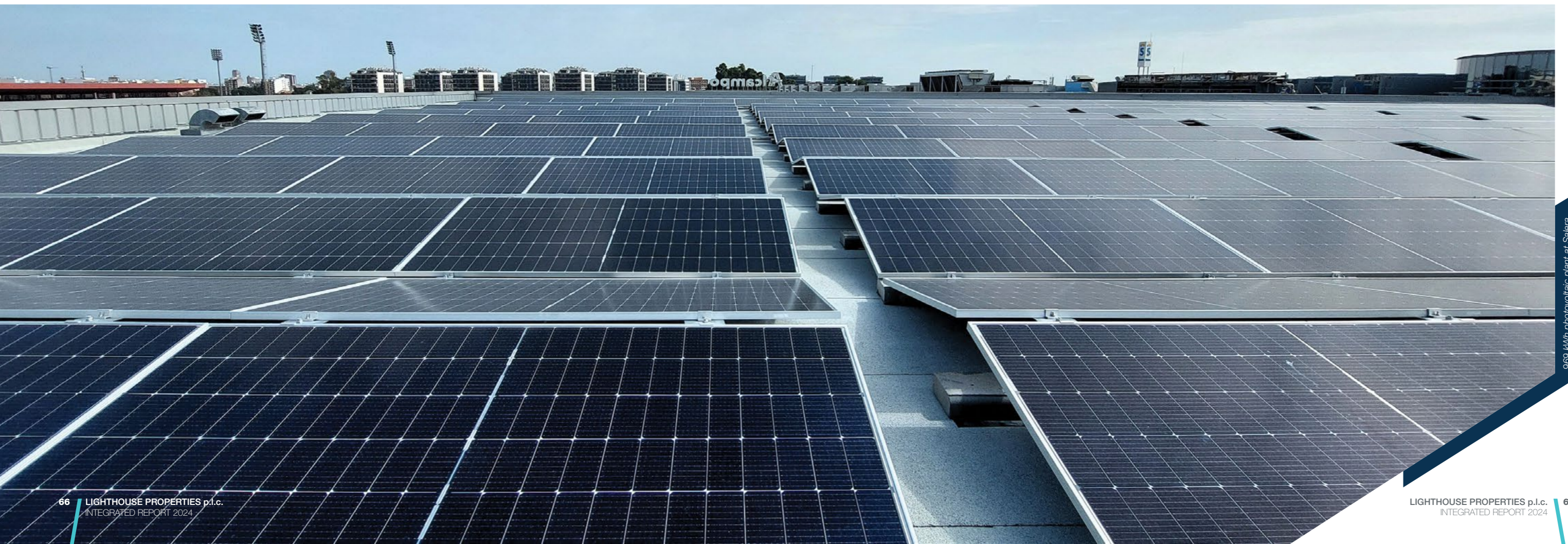
969 kWh photovoltaic plant at Salera
