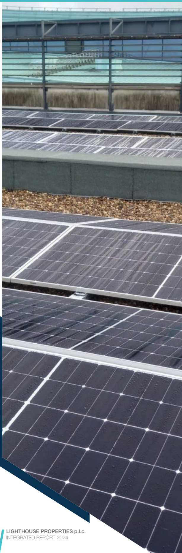
PV Installation at Forum Coimbra
