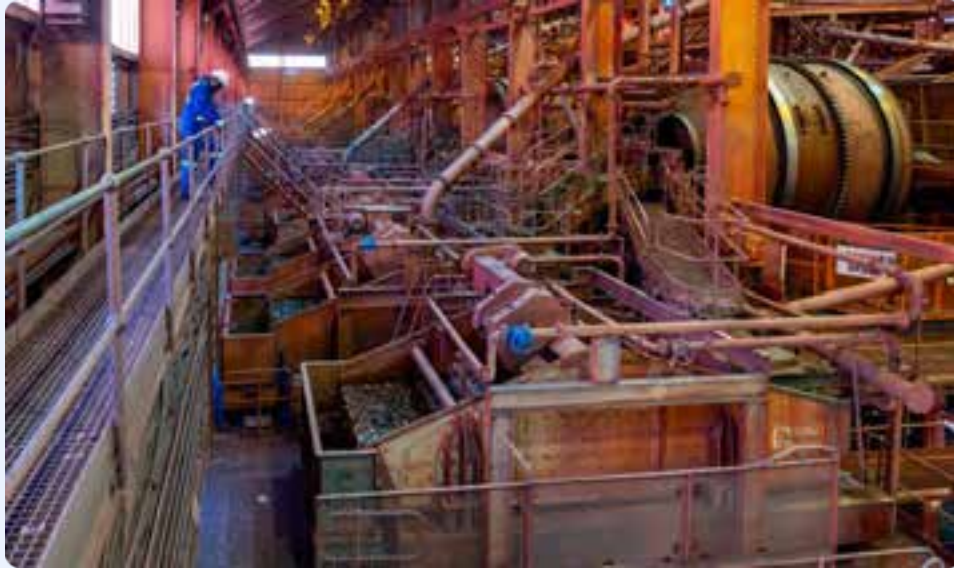
Dense media separation (DMS) processing plant at Sishen, with the current DMS drums to be upgraded as part of ultra high dense media separation (UHDMS) technology project.
