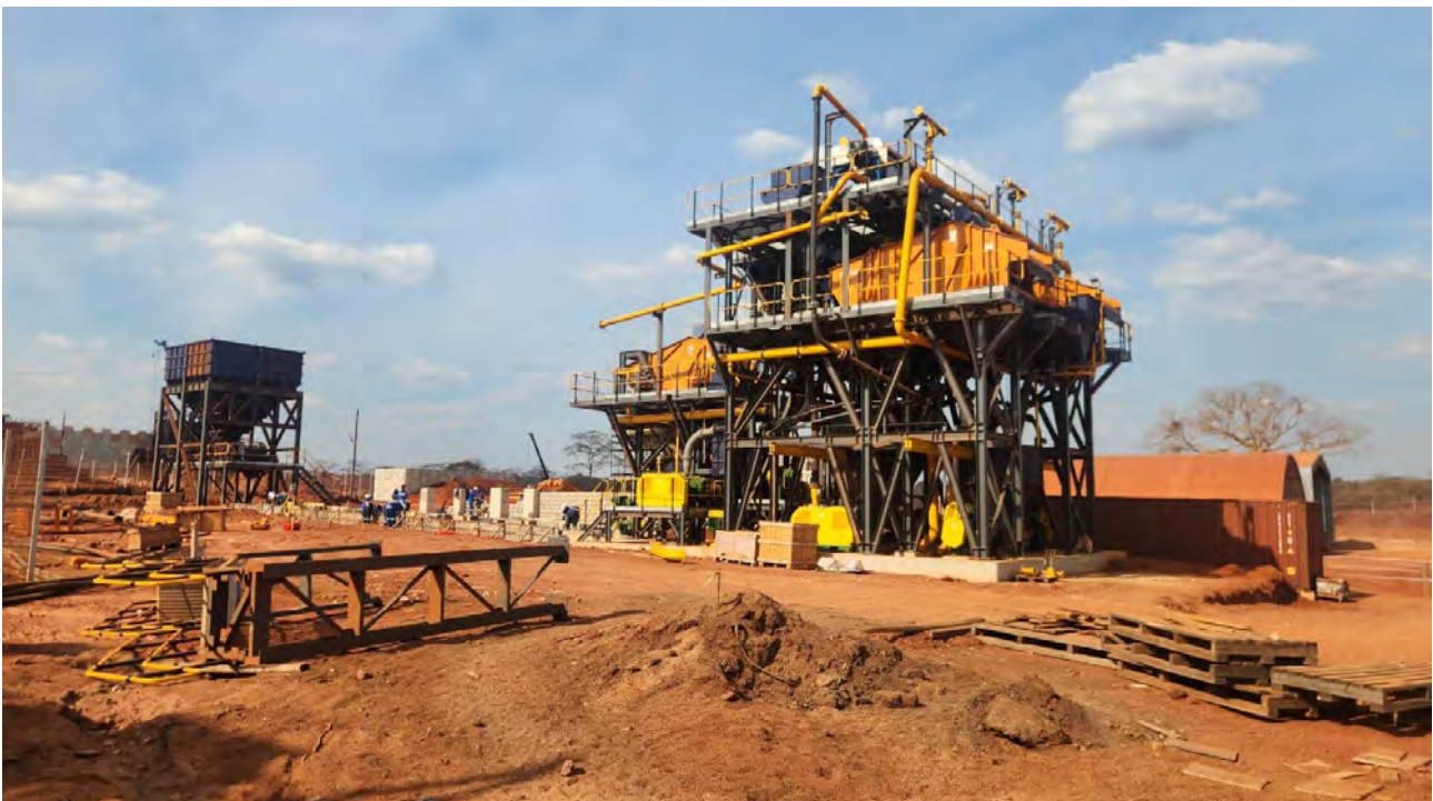
Above: Part of the construction for MRM's second processing plant, as seen in early September 2024
