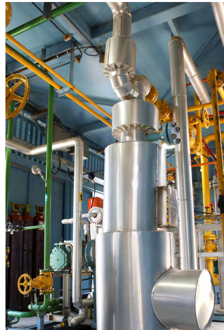
Mixed refrigerant loading manifold.
