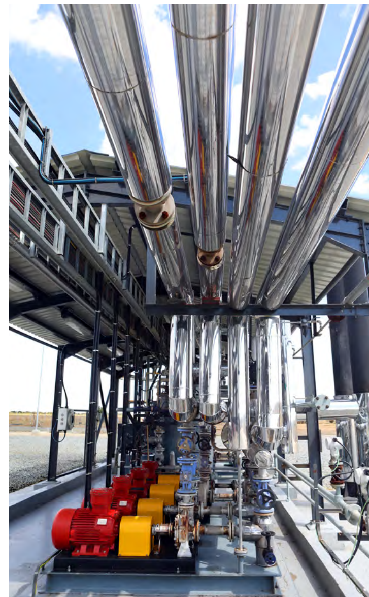
Conduction oil pumps.
